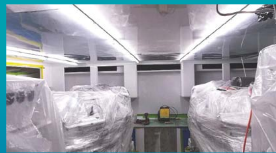
Protected from sanding dust and overspray in the Weaver Boat Works shop, the Weaver 80's twin MTU 16V2000 M93 diesels are rated at 2400 hp each. Photo by Weaver Boat Works
